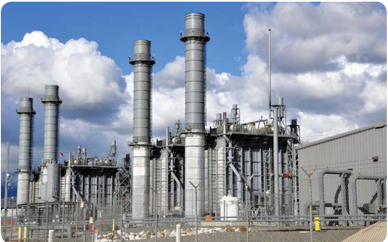
A single control platform was required that would have to interoperate with different types of signals and communication protocols
