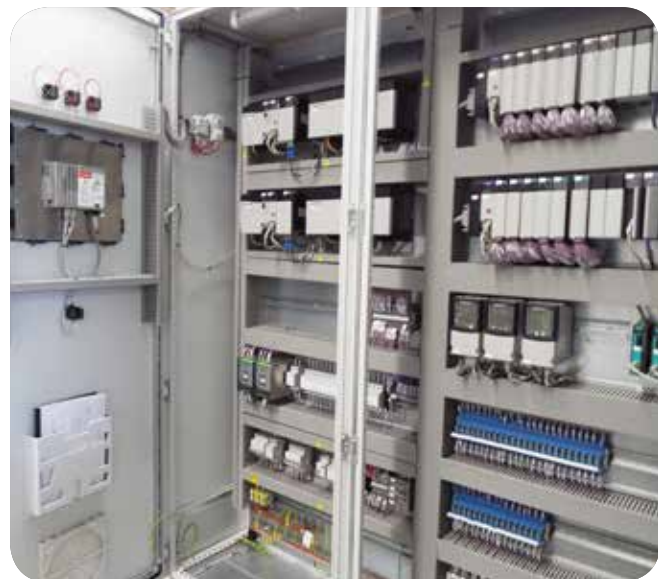
The compressors are automated using high-level process controllers, in redundant configuration
