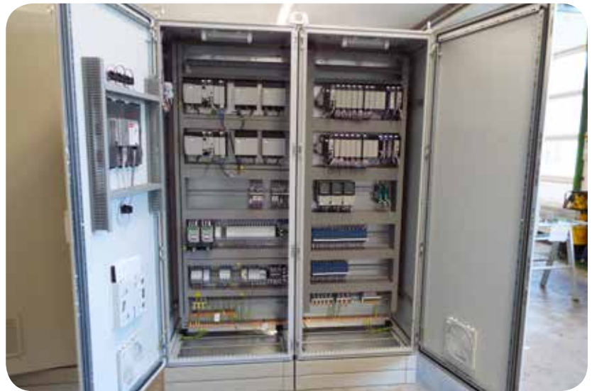
The primary requirements were for a control solution that would deliver high reactivity, integration and reliability
